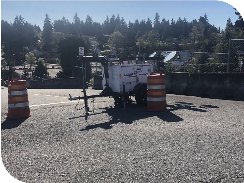
Diesel-powered temporary light plant
